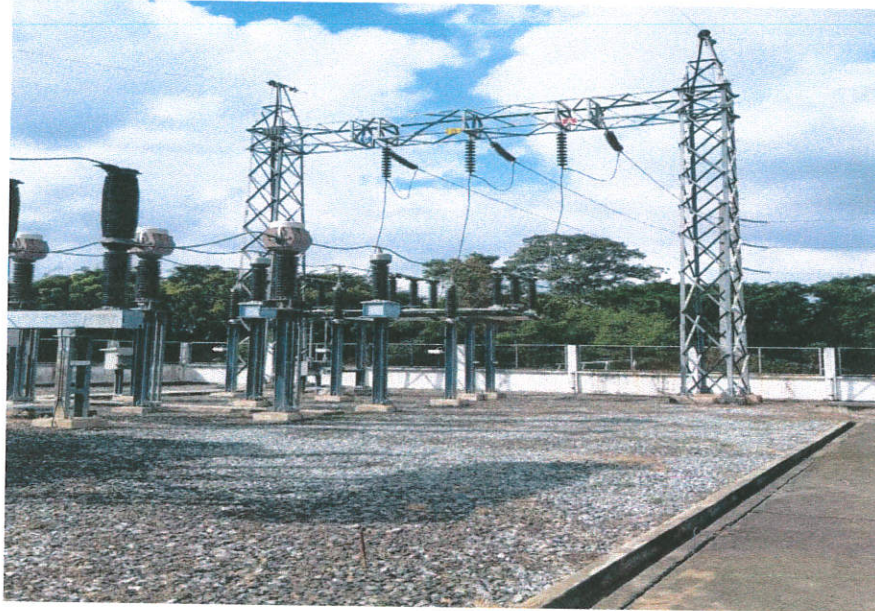
SUB STATION 115 kV
